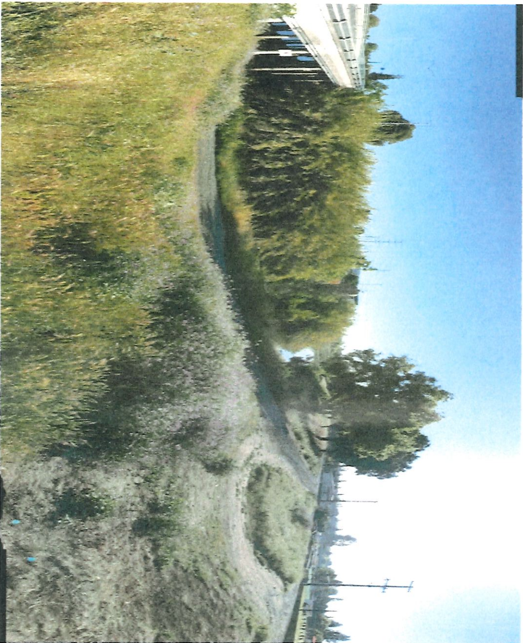
Picture # 20 Pershing bridge Looking upstream or easterly of the Calaveras River channel.
